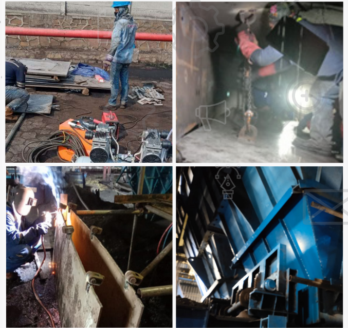
JASA REHABILITASI LANE BELT FEEDER A & B COAL HANDLING PT PLN Indonesia Power UBP Suralaya
