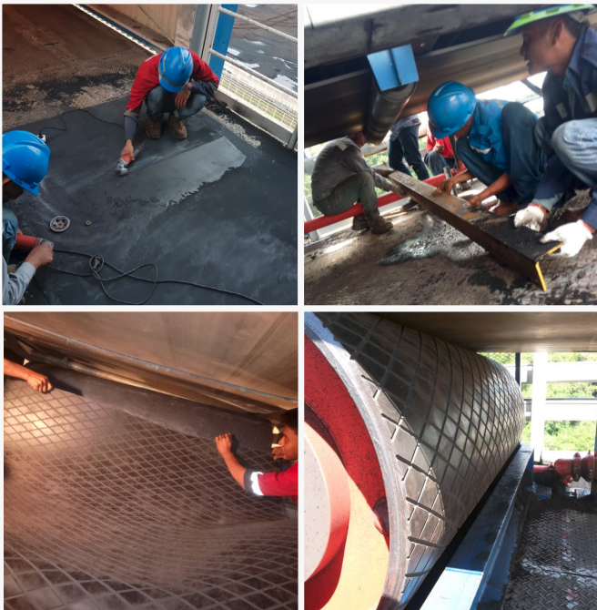
RELAGGING PULLEY PT Lestari Banten Energi
